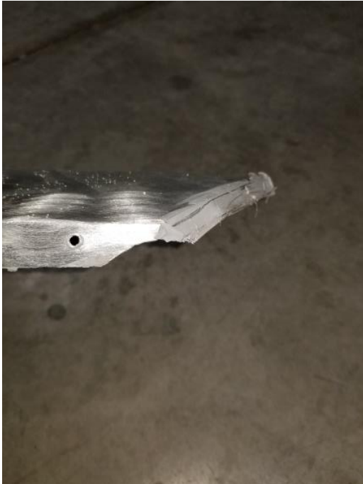
Photo 17- Aluminum cap flashing notched for retaining frame the end of the cap flashing also curled closed against the retaining frame.
