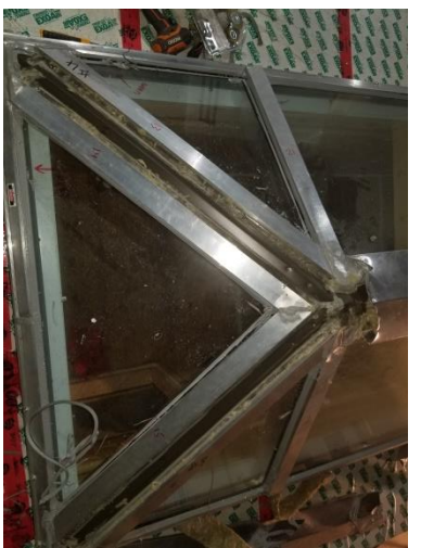
Photo 15- Aluminum closure panels at apex corner rafters and ridge rafters, riveted in place with joints sealed with silicone.
