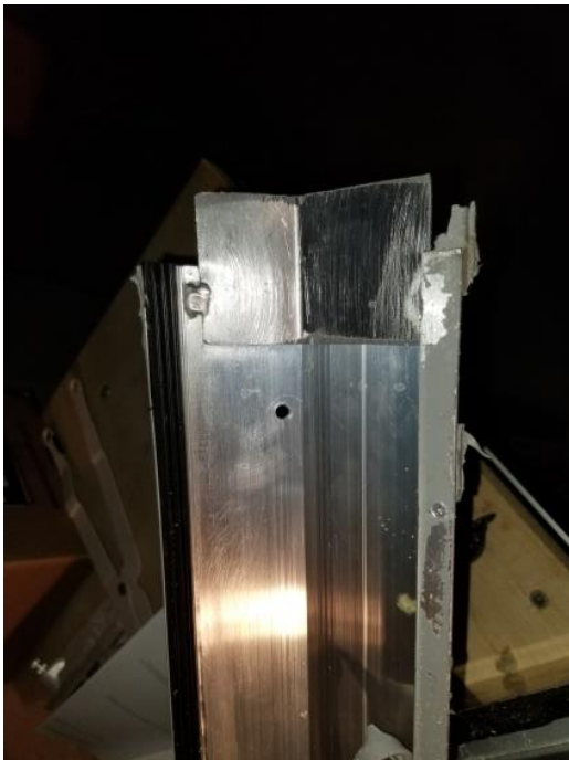
Photo 19- Formed 18 ga aluminum tab on backside of retainer frame at butt joints.
