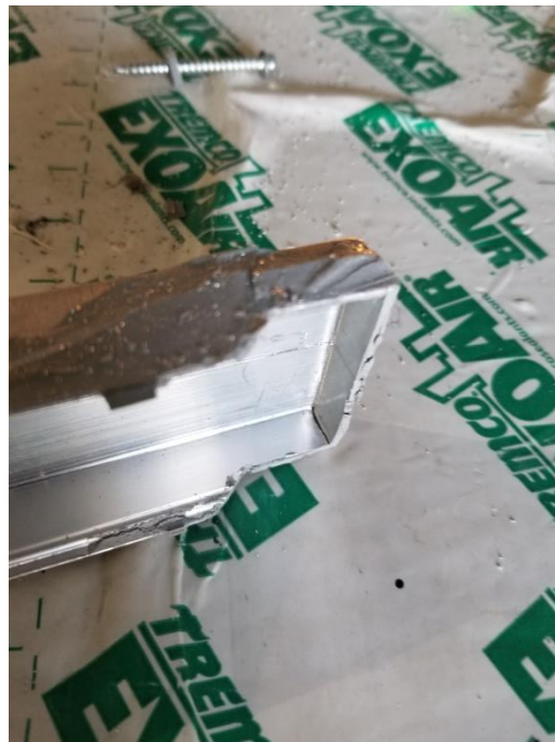
Photo 20- Aluminum trim cap notched and curled closed at retaining frame end.
