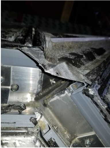
Photo 10- Intersecting sides of the ridge rafters and the end rafters were welded together along the outside edge of the corner joint
