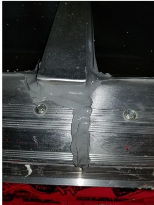
Photo 18- Aluminum trim cap curled closed against the retaining frame, sealed to retaining frame and glazing with silicone. Retaining butt joint also sealed with cap bead of silicone.
